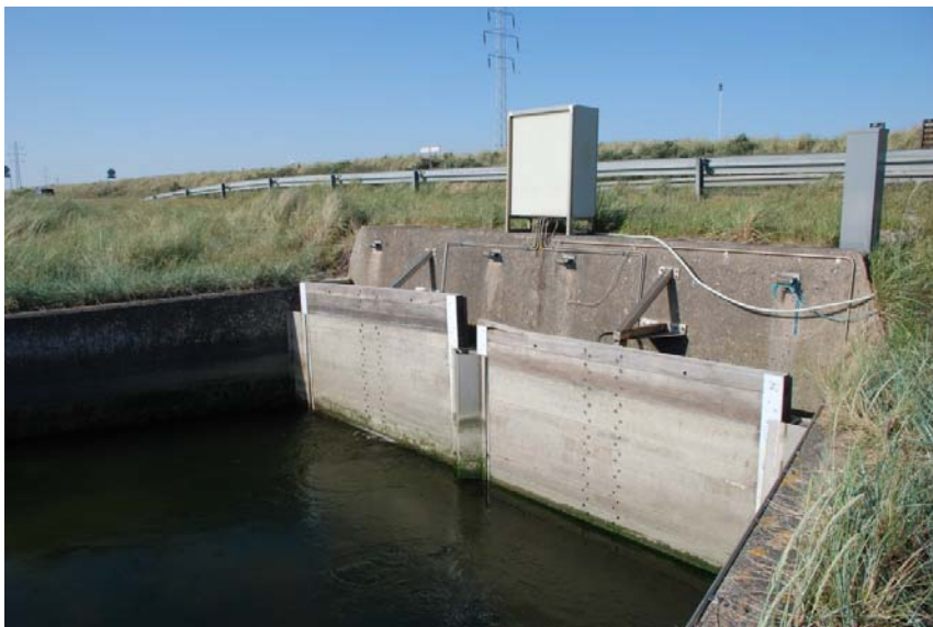
The automatic sluice gate at Harboøre Tange
